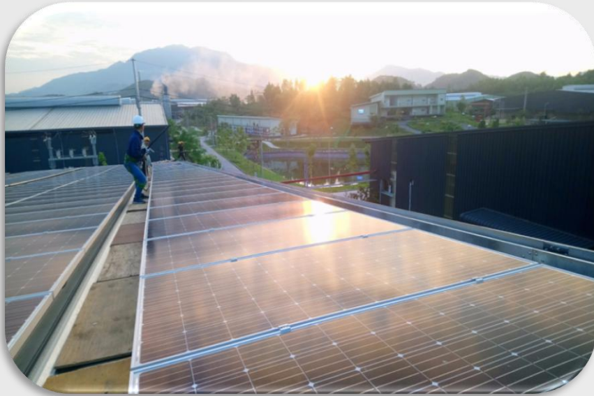
1MW Roof Project Vietnam Year 2019
