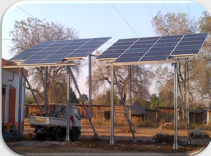
500kw Solar Power PV Station Mozambique year 2015
