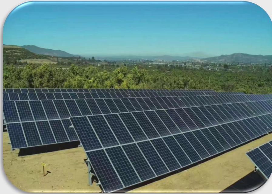
2MW Power Plant Thailand year 2012
