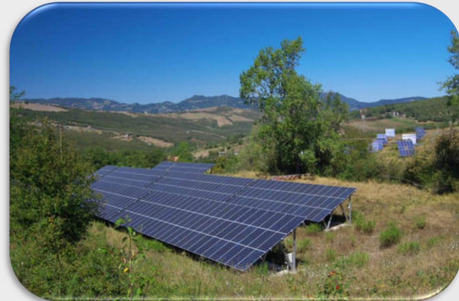
500kw Power Plant Italy year 2018
