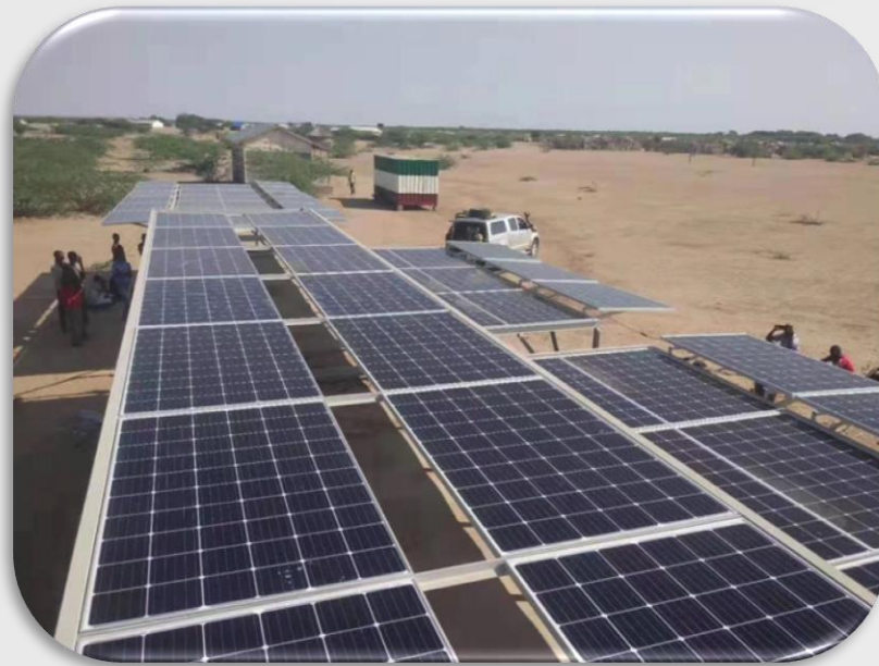
1MW Solar Power PV Station Kenya year 2015
