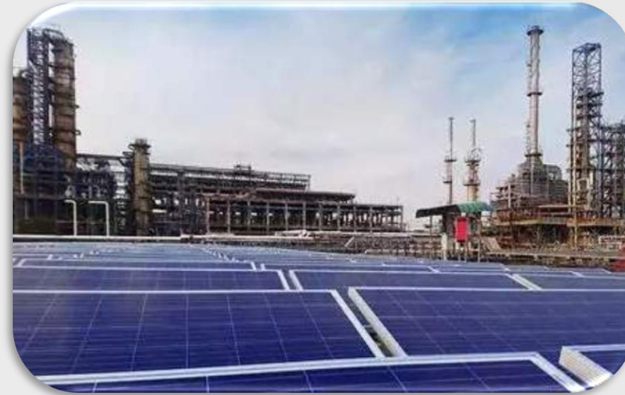
5MW Power Plant India year 2018
