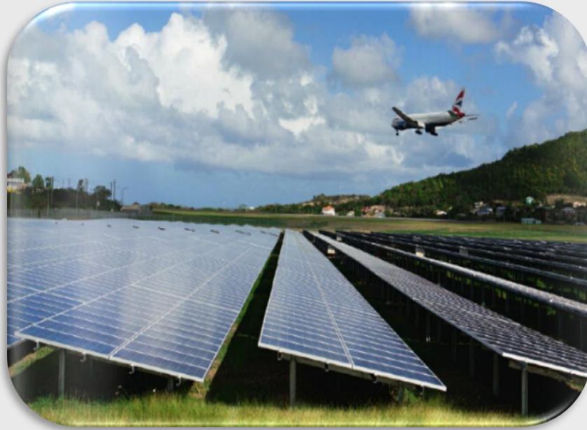
3MW Solar Power PV Station Antigua year 2016
