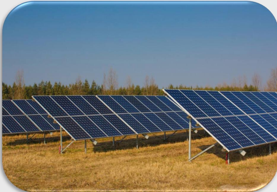
3.5MW Solar Power PV Station Czech year 2016
