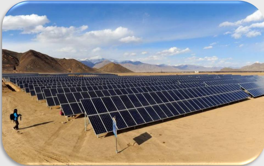
15MW Power Plant Brazil year 2017
