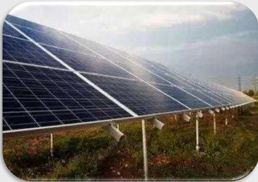
5MW Power Plant France year 2012
