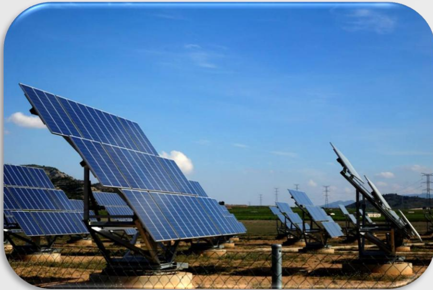
2.8MW Power Plant Spain year 2012
