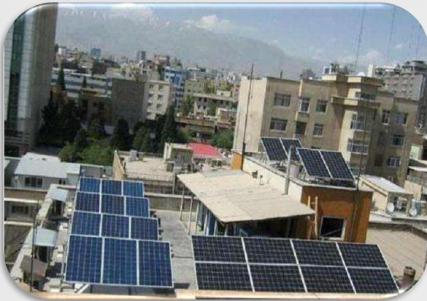
300kw roof system Iran year 2015
