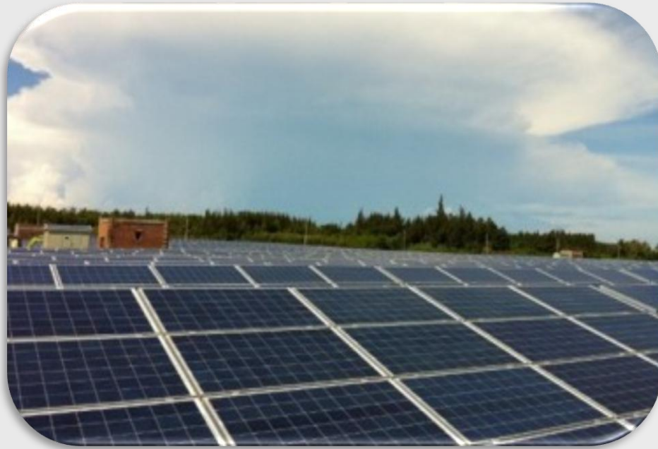
2MW On-grid Solar Power Project Malaysia year 2014
