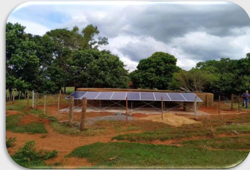
200kw Ground Project Philippine year 2016
