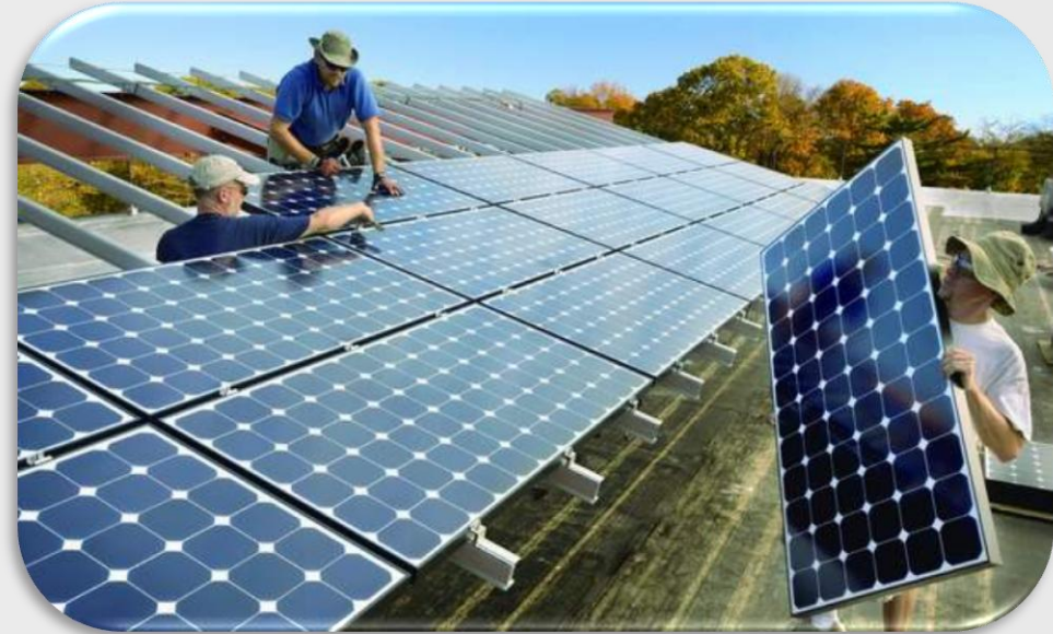
800kw Power Plant Chile year 2016
