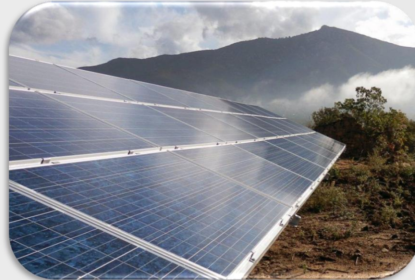
4.5MW Solar Power PV Station Corsica 2014
