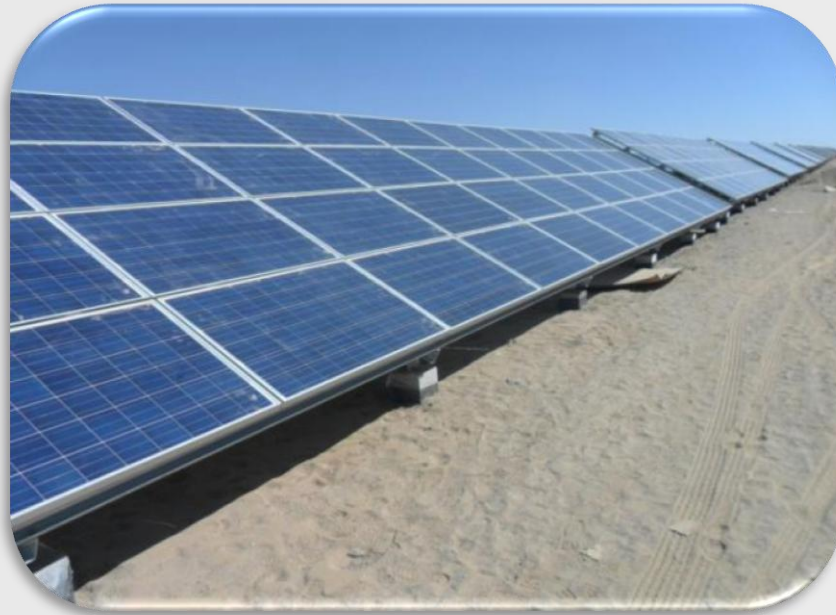
30MW Ground PV Station Qinghai Province China year 2011
