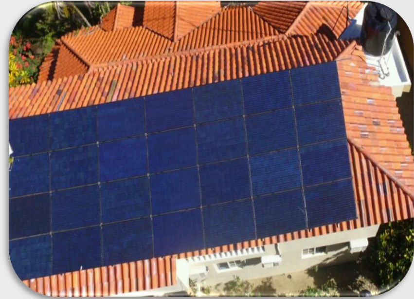
500KW Solar Power PV Station Dominica year 2016
