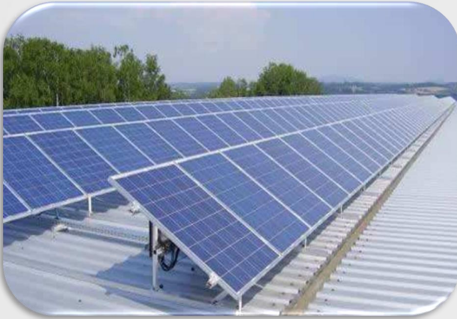
3MW Solar Power Plant Hungary year 2019
