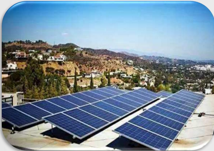
500kw Power Plant Egypt year 2017
