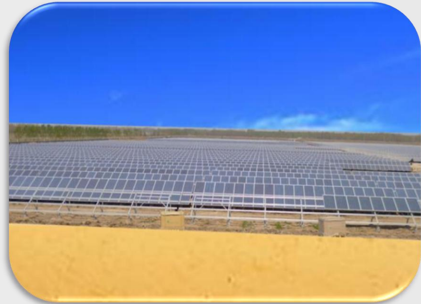
20MW SUMEC Xuzhou Solar Power PV Station Jiangsu Province China year 2012
