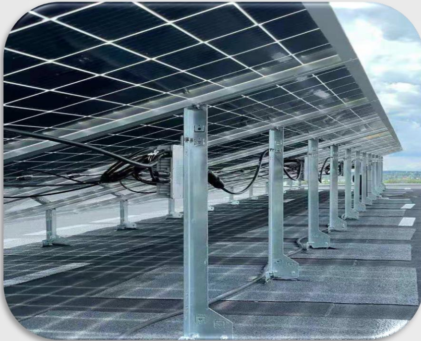
200KW solar system Finland year 2021
