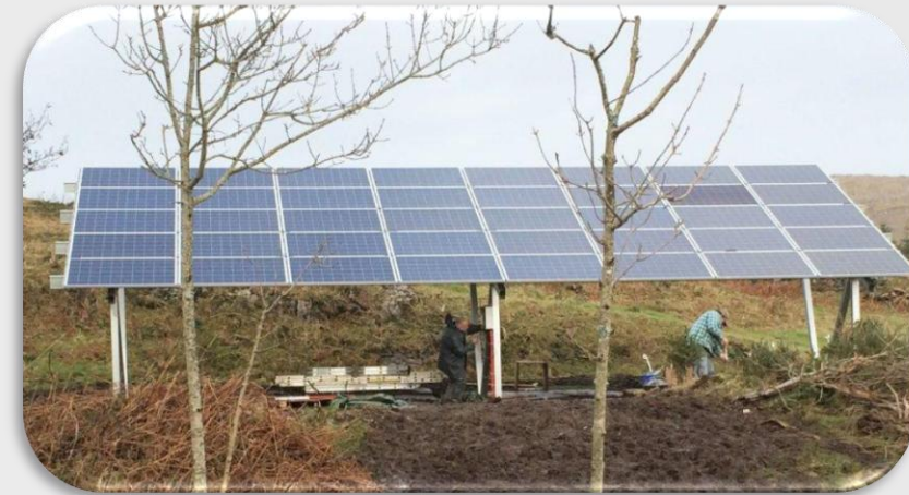
100KW Solar System Cork 2018
