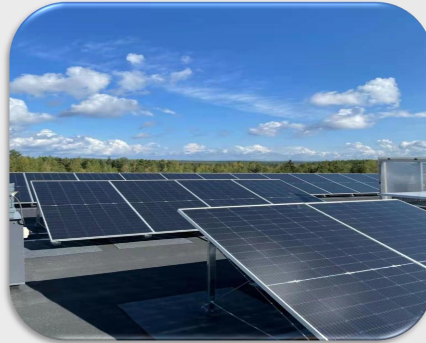
300kw solar system Finland year 2021
