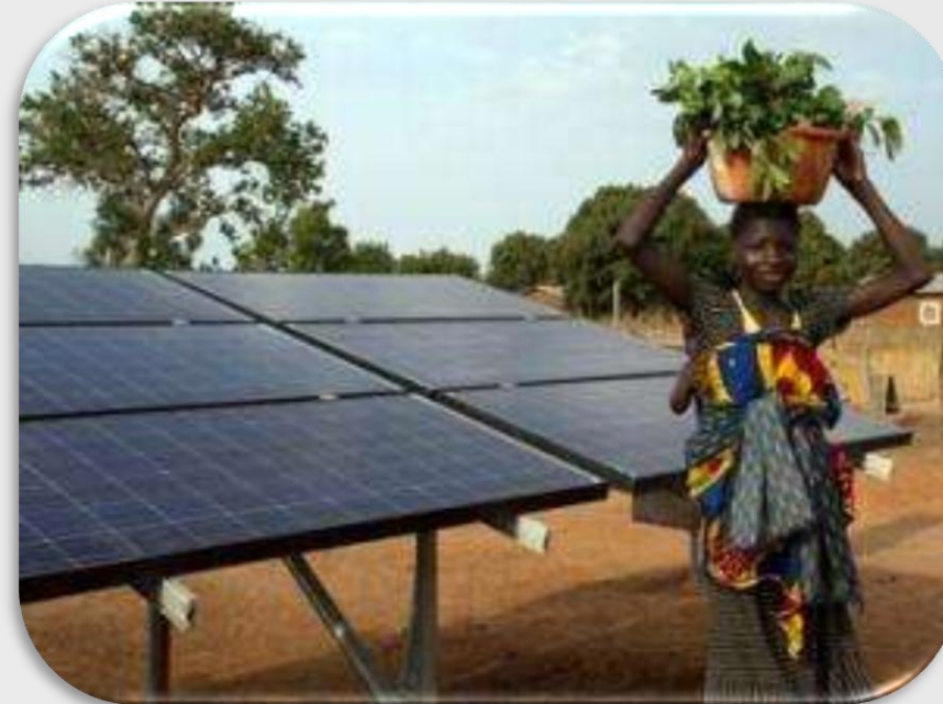
200kw Solar System Nigeria year 2018
